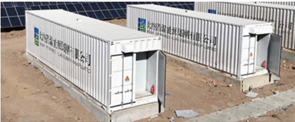
Figure 2-2: Image of a typical container housing the battery storage modules
