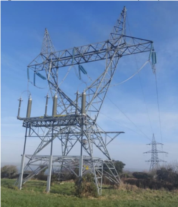
Figure 2-9: Line Cable Interface Mast (LCIM)
